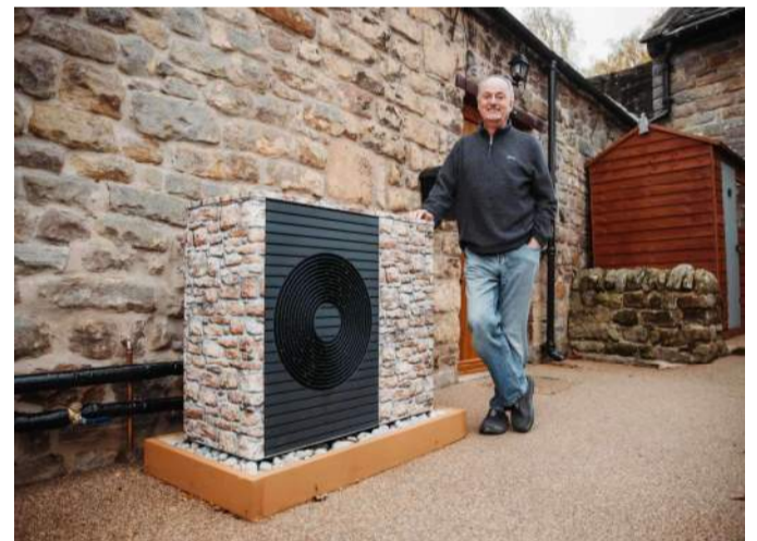
External (disguised!) heat pump unit
